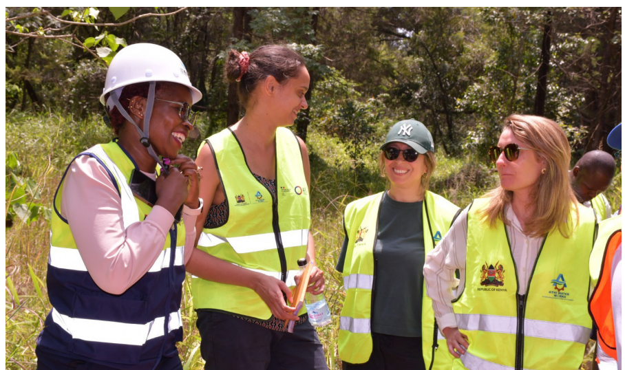
Infrastructure in Harmony with Nature . Eng. Bonnie Nyadwaro, Anne-Sophie Triboulet, Fariza Chalal, and Melanie Grignon during a site visit at Karura Forest, overseeing the Gigiri-Karura transmission pipeline while ensuring strict environmental and social safeguards.
